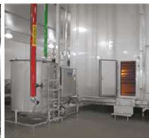
Full recirculating cleaning system
